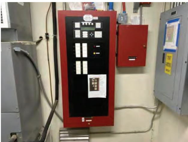
35 - FIRE ALARM PANEL
