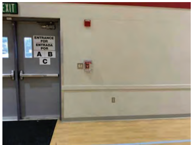
36 - FIRE ALARM SYSTEM
