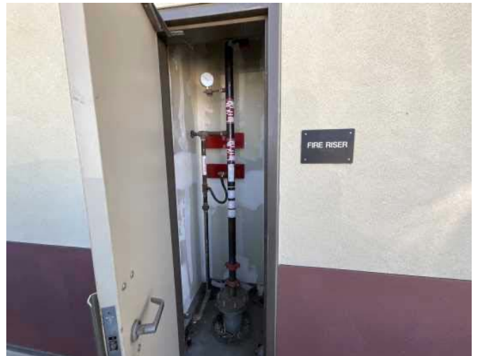
22 - FIRE SUPPRESSION SYSTEM
