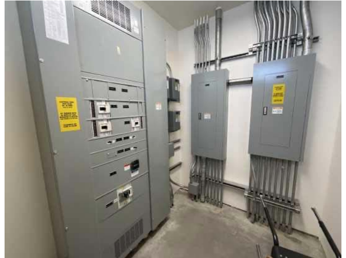
20 - MAIN ELETRICAL EQUIPMENT
