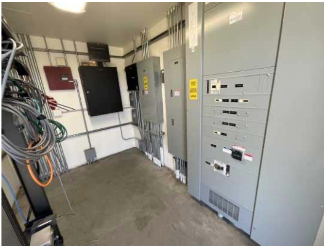
21 - MAIN ELETRICAL EQUIPMENT
