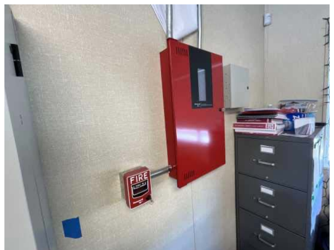
24 - FIRE ALARM PANEL
