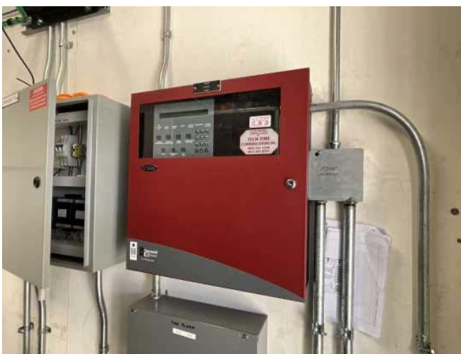
23 - FIRE ALARM PANEL
