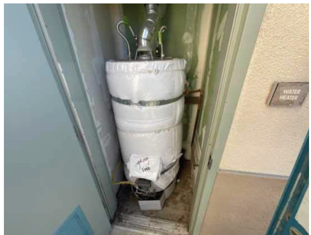
12 - GAS WATER HEATER
