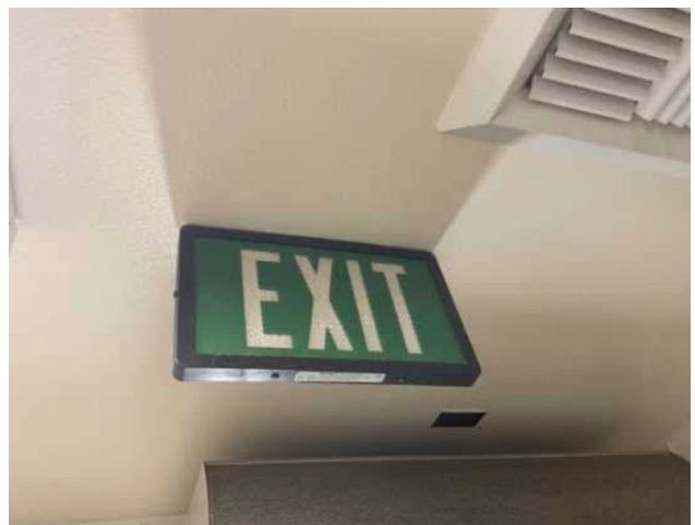
24 - EMERGENCY AND EXIT LIGHTING
