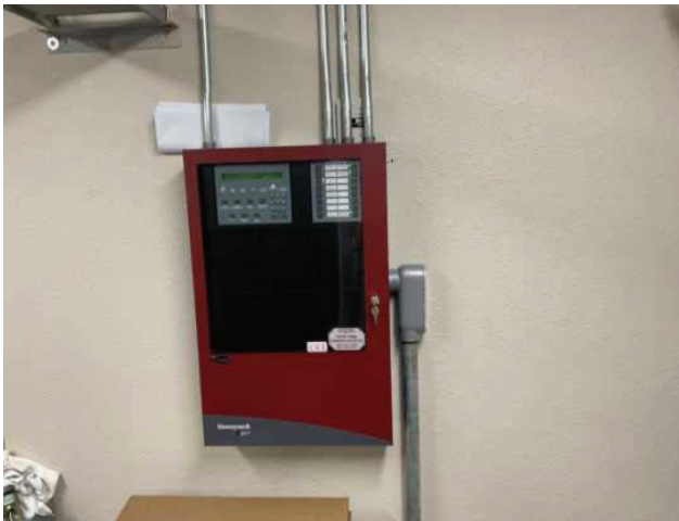
27 - FIRE ALARM PANEL
