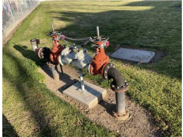
20 - FIRE SUPPRESSION BACKFLOW PREVENTER
