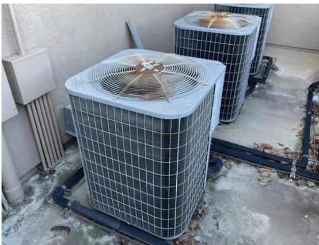
17 - SPLIT SYSTEM CONDENSING UNITS
