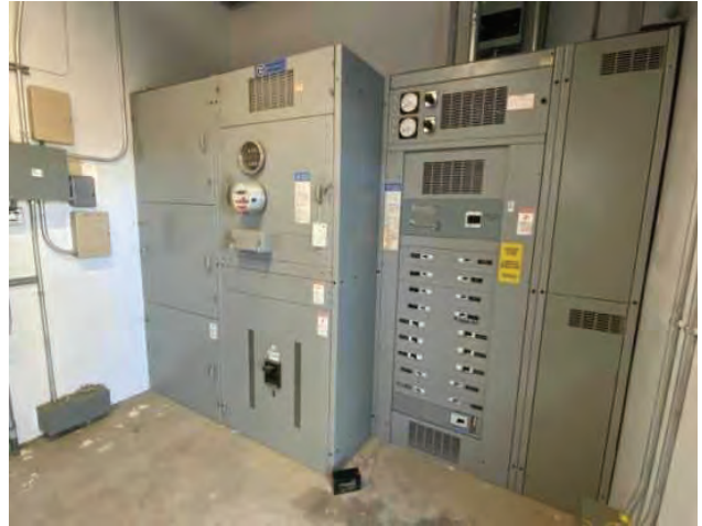
32 - MAIN ELETRICAL EQUIPMENT
