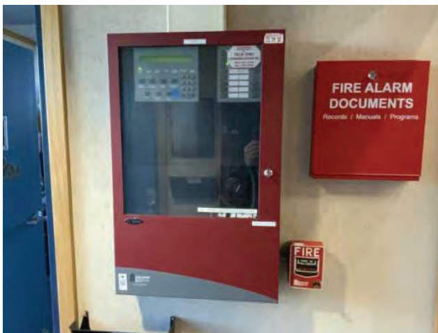
35 - FIRE ALARM PANEL
