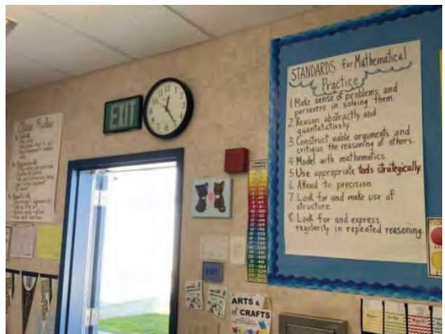
36 - FIRE ALARM SYSTEM
