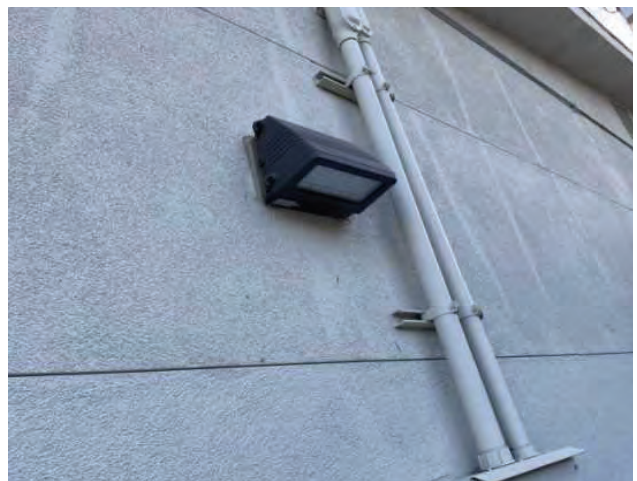
24 - LED EXTERIOR FIXTURES
