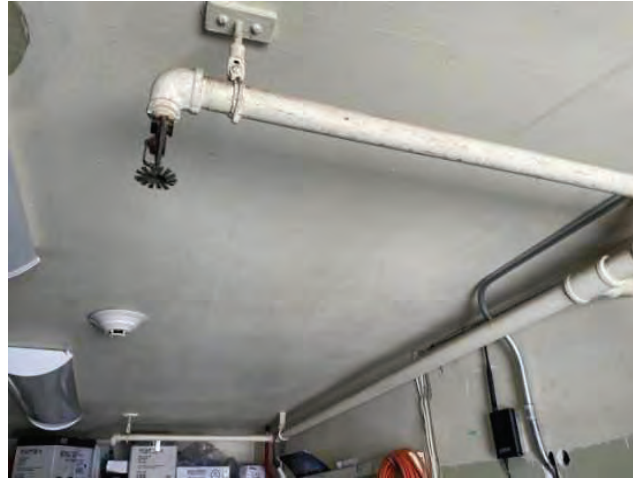
20 - FIRE SUPPRESSION SYSTEM
