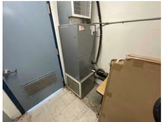
16 - SPLIT SYSTEM FCU
