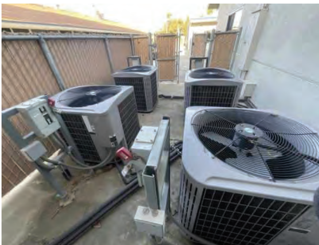
17 - SPLIT SYSTEM CONDENSING UNITS
