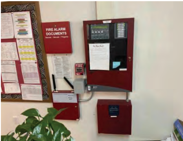
21 - FIRE ALARM PANEL
