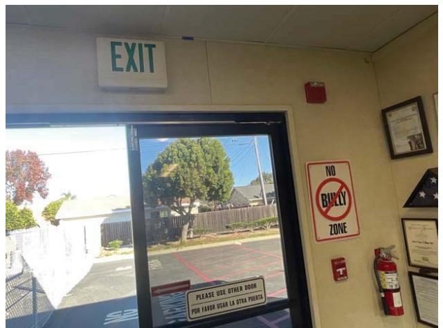
18 – FIRE ALARM SYSTEM
