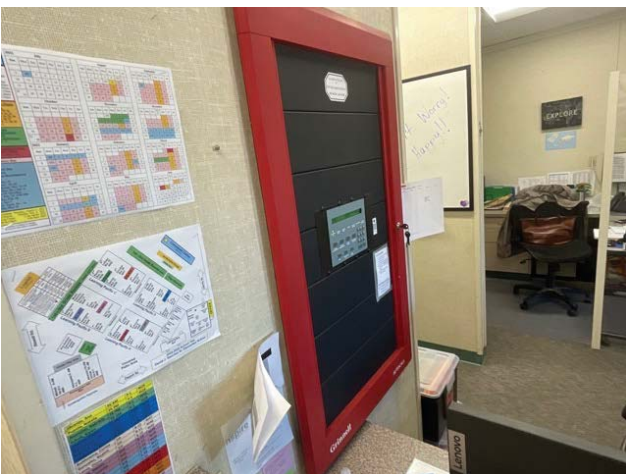
17 – FIRE ALARM PANEL
