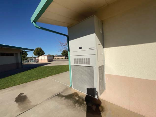
13 – WALL MOUNTED PACKAGED UNIT
