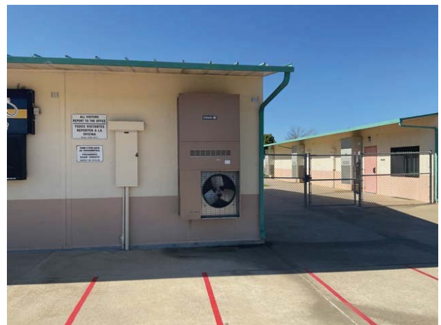
12 – WALL MOUNTED PACKAGED UNIT
