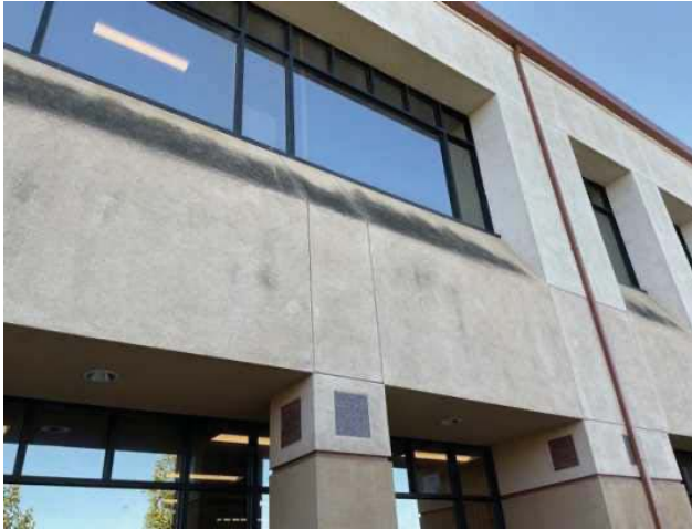
25 - MILDEW PRESENT ON EXTERIOR WALLS
