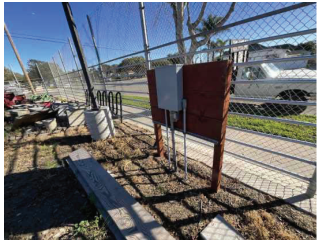
22 - MAIN ELECTRICAL EQUIPMENT
