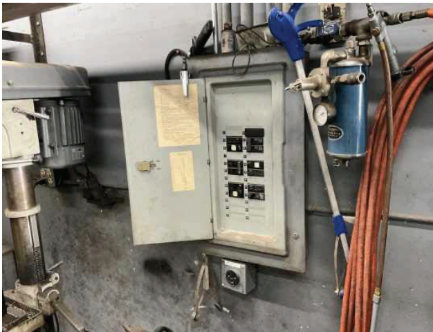
21 - MAIN ELECTRICAL EQUIPMENT
