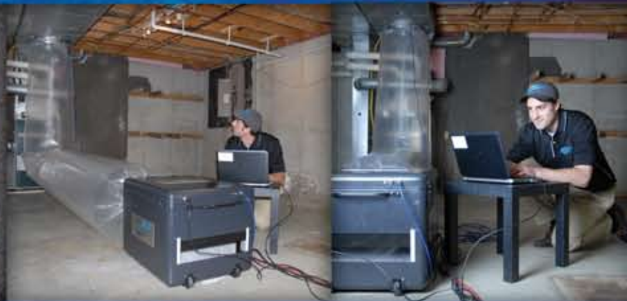
A professional AeroSeal technician will monitor the duct leakage in your home
