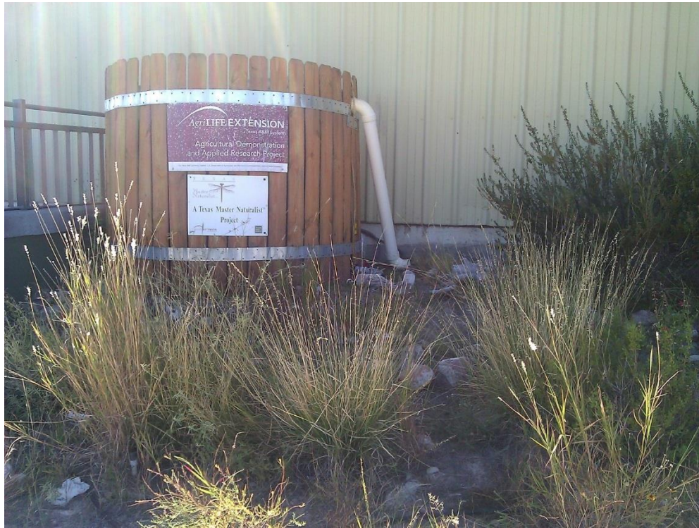
Figure 11-4 Rainwater Harvesting System used to Irrigate Xeriscape
