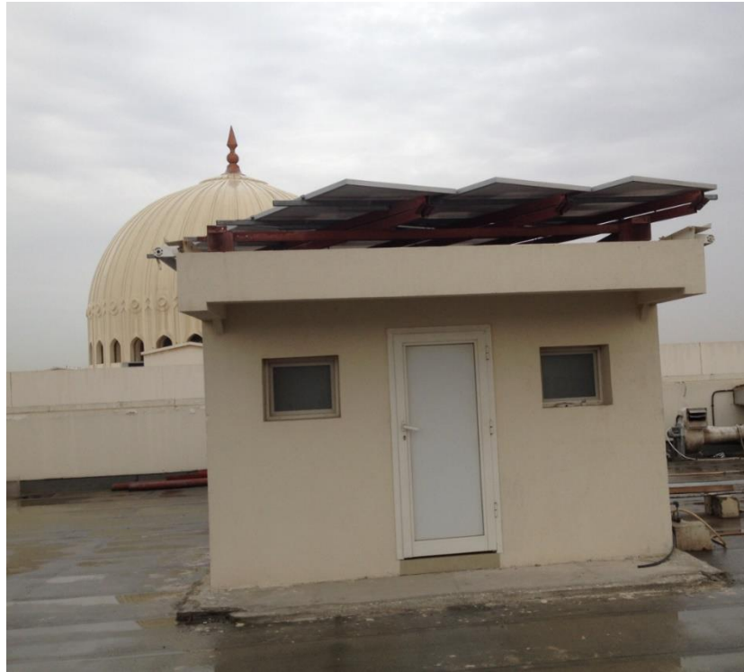
Figure 20: Solar PV for Efficient Building – 1.5 kW
