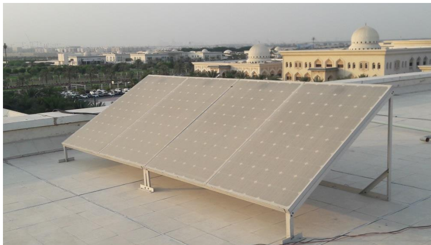
Figure 21: Solar PV Panels
