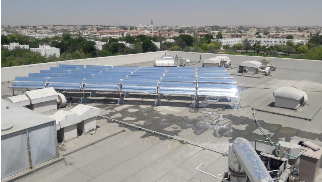
Figure 18: 10 Tones (35 kW) Solar Air Conditioning System
