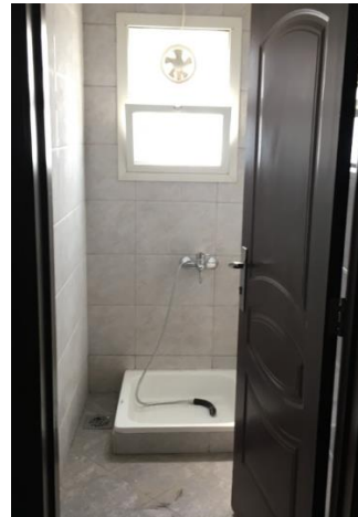
Picture of a shower room in student dormitory whose water is supplied to grey water system (Example: University of Sharjah)
