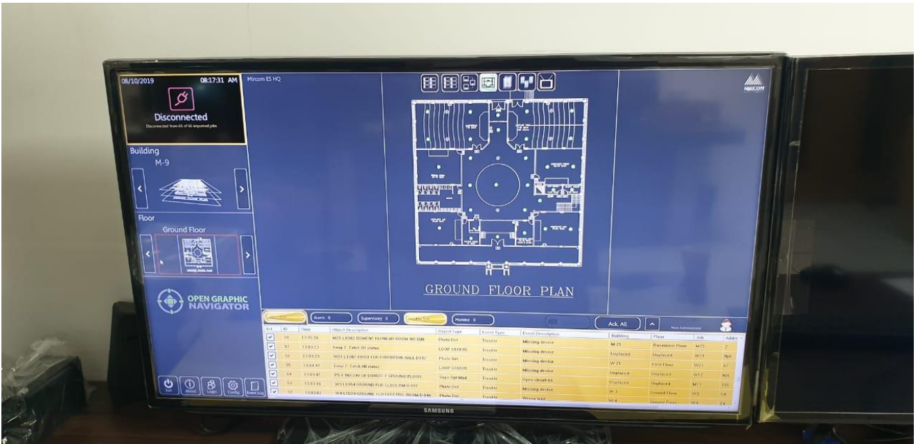
Figure 14: A screen showing the ground floor of one building with the locations of sensors
