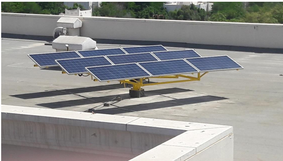
Figure 19: Solar PV (3 kW)
