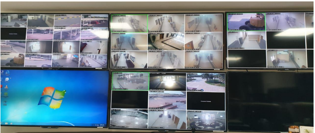
Figure 12: Several screens showing the operation of the new Building Monitoring System
