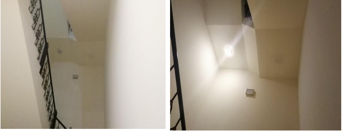
Figure 17: Motion sensors for lighting
