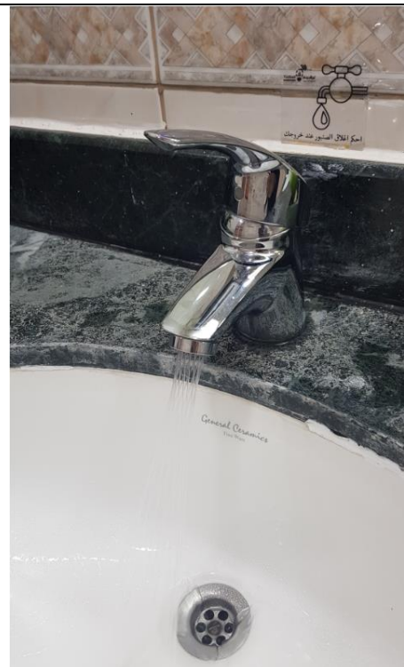
Example of efficient water faucet (low flow type) (Photo source: University of Sharjah)
