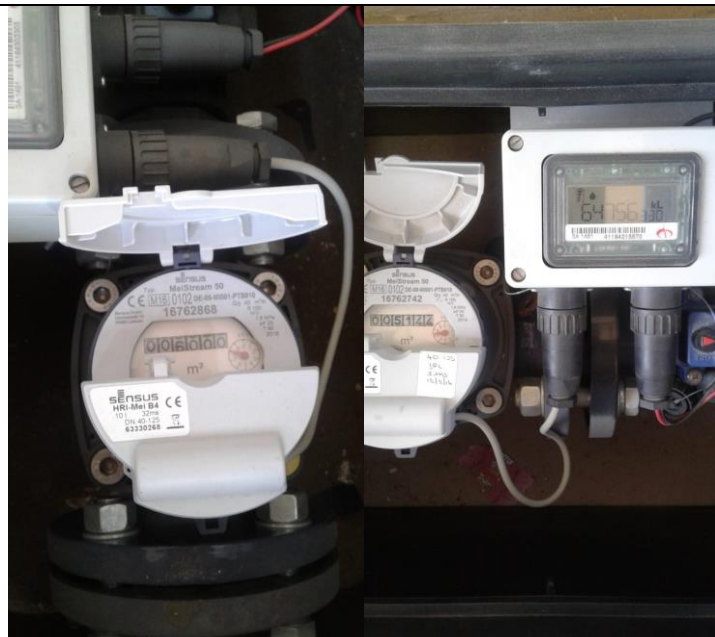
Installation of Smart water meters (Photo source: University of Sharjah ) to monitor the use, detect leaks and conserve water
