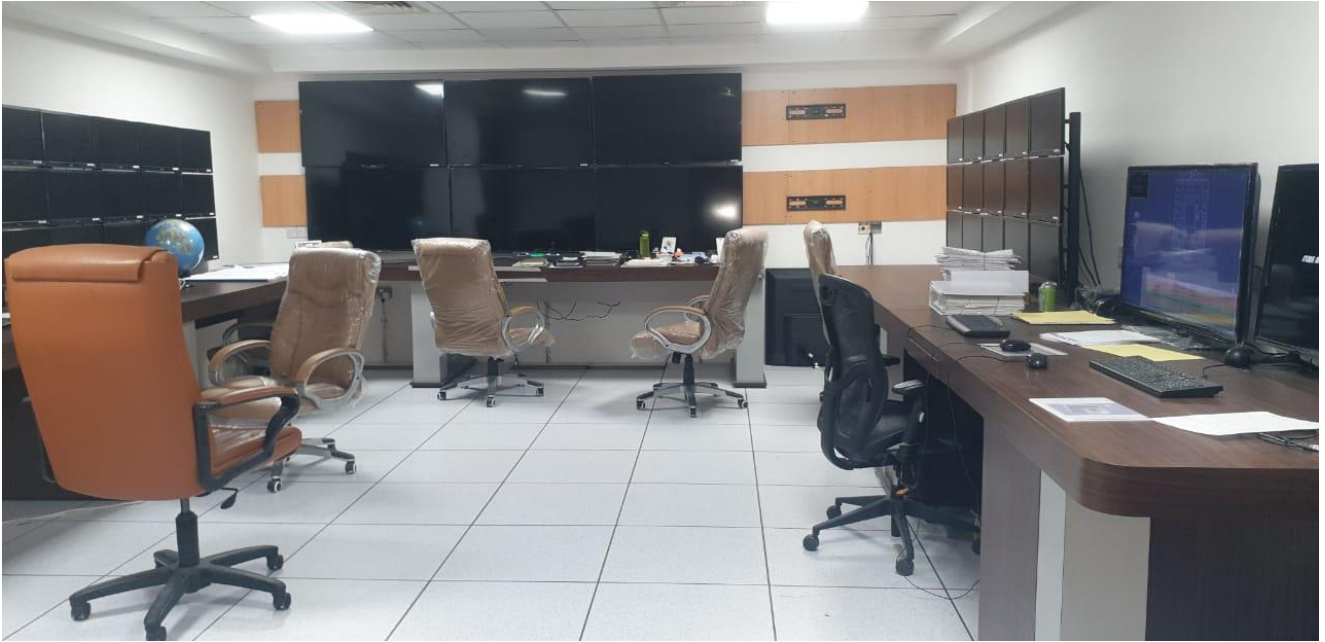
Figure 11: Control room of Building Monitoring System
