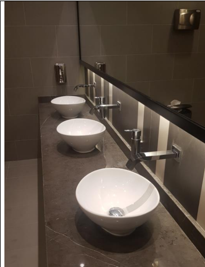
Example of efficient water faucet (automatic type) (Photo source: University of Sharjah )
