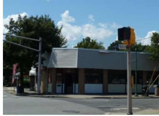
P-B3b. The city should encourage facade and sign improvements on Campbell Ave. For example, the roof structure on the building pictured above hides original architectural details and makes the business appear shuttered.
