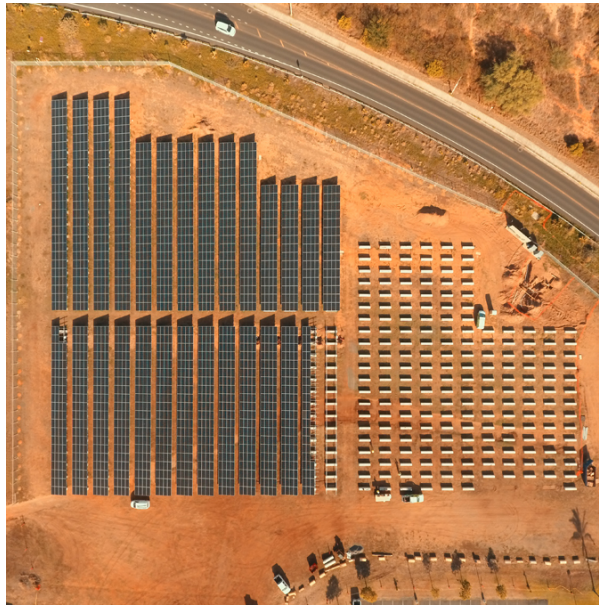
Photovoltaic panels at UH Maui College.
