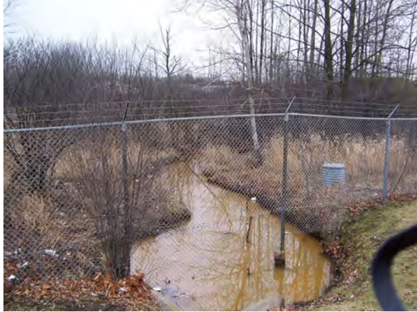
Figure 3-11 - Downstream area where backups occur that flood the Maintenance and Materials Building parking lot
