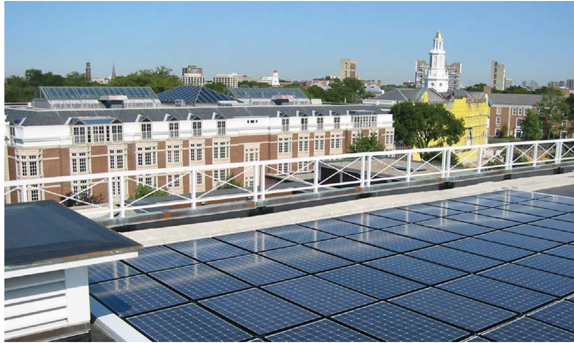
Harvard Business School recently installed 172 solar photovoltaic panels which will supplant the emission of about 75,000 pounds of carbon monoxide annually -- the equivalent of about 220 fewer cars on the road each year.
