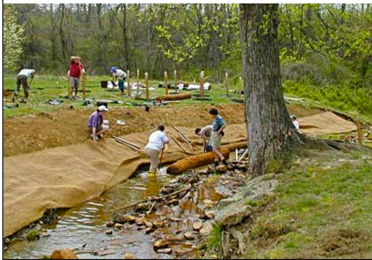
Figure 35 A riparian buffer can also be constructed out of engineered materials as shown here.
