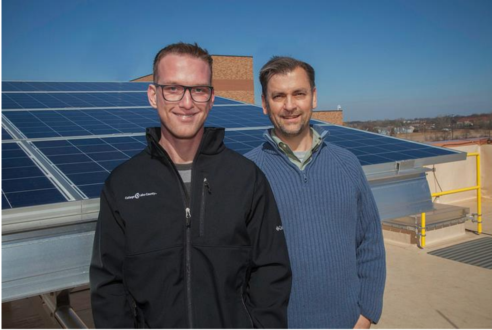
Solar PV Panels on Science Building
