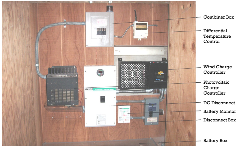
Figure 3 - Wiring inside the Strawbale House
