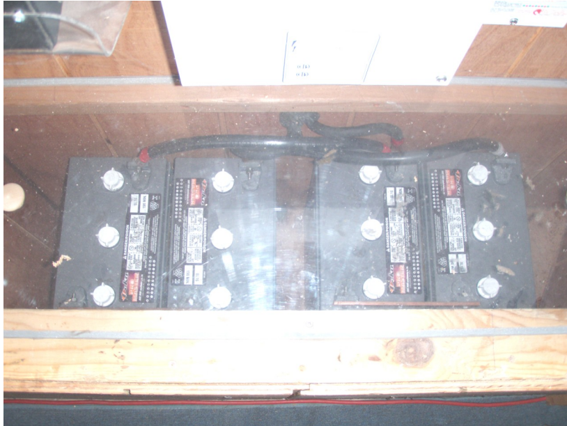
Figure 12 - Strawbale Battery Bank
