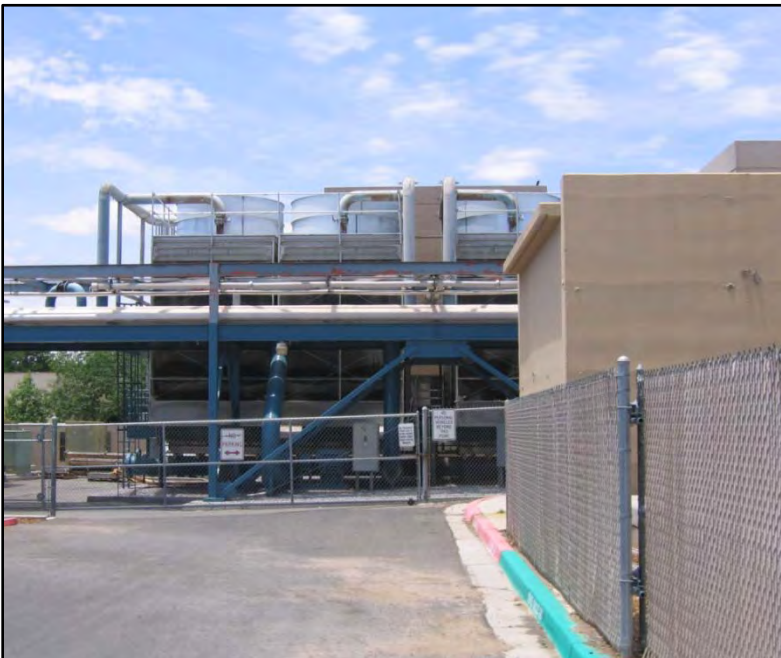
Figure 11. Cooling Towers behind Central Plant (NG-Fired Turbines are within Building on the Right Side).
