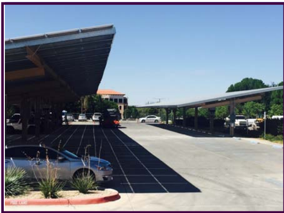
Solar covered parking in Lot 100
