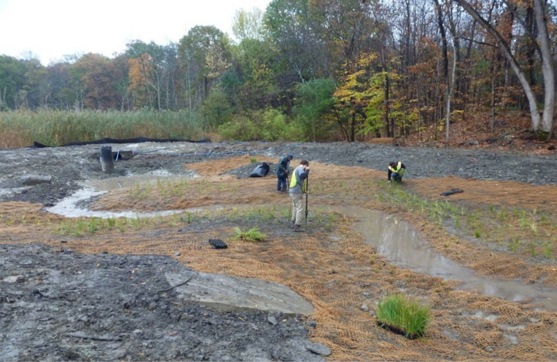
THE CONSTRUCTED WETLAND BEING PLANTED WITH THOUSANDS OF WETLAND SEDGES, GRASSES AND HERBACEOUS PLANT PLUGS OCTOBER 2014
