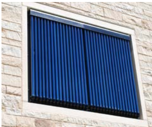
Solar thermal panel creates domestic hot water for immediate use
