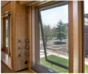
Naturally ventilated space at Kroon Hall
