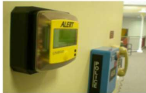
Figure 1: Installed Alert Beacon
