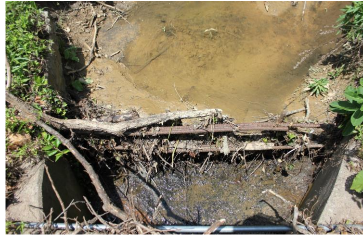
Partially Clogged Trash Screen Upstream of Culvert Entrance
