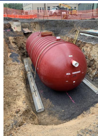
Runoff Capture and Reuse / Rainwater Harvesting
