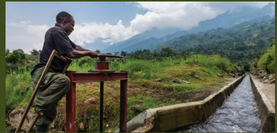
The Mutsora run-of-the-river mini hydroelectric facility is located just outside the Virunga National Park, North Kivu. Photo Credit: Brent Stirton/Getty Images.
