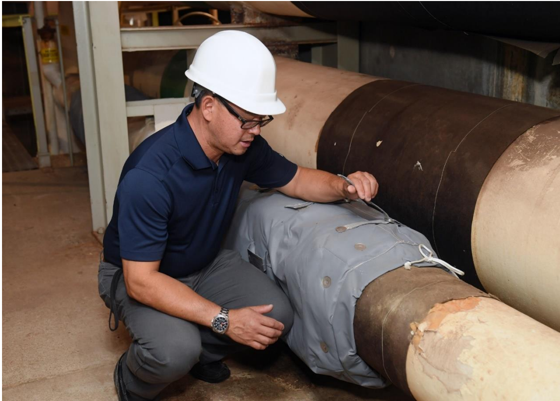
Figure 1.3 Steam Pipe Insulation saves energy from steam distribution system.
