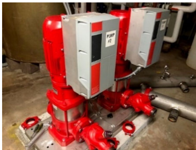
Figure 1.2. Booster pumps with variable speed drives installed at the LSC.
