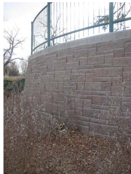
The retaining wall at the College Ave. underpass is a good example of a rectangular, flat face concrete block structure.
