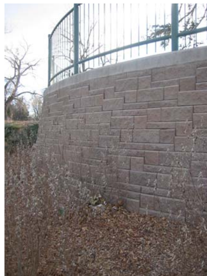
The retaining wall at the College Ave. underpass is a good example of a rectangular, flat face concrete block structure
