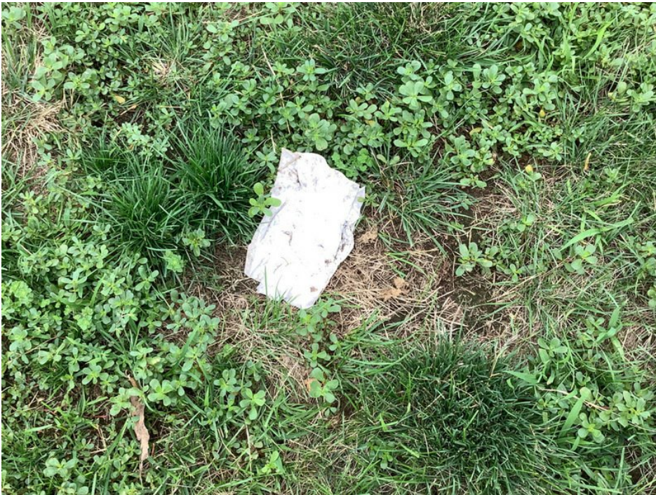
View of trash on the northwest section of the green roof.
