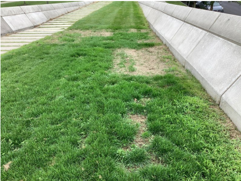
View of dead vegetation on the northwest section of the green roof (facing west).
