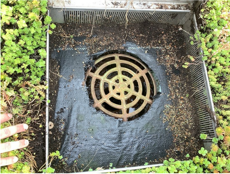
View of accumulated sediment in a roof drain on the northeast end of the green roof.
