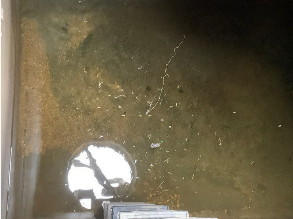
View of accumulated sediment in the east side of the sand filter.
