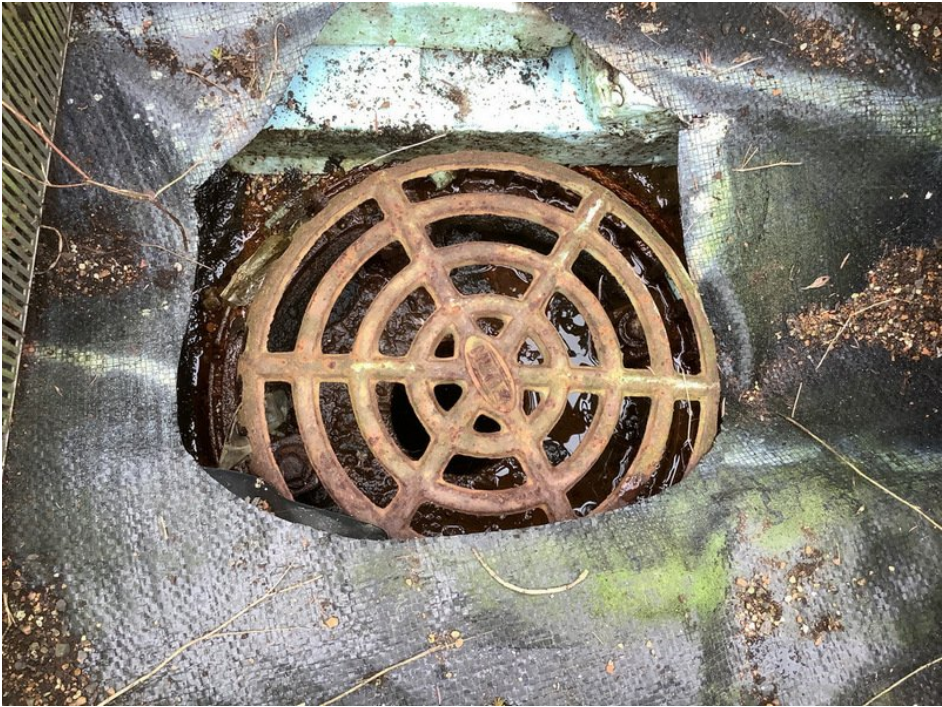
View of a minor amount of accumulated sediment in a roof drain on the north end of the green roof.
