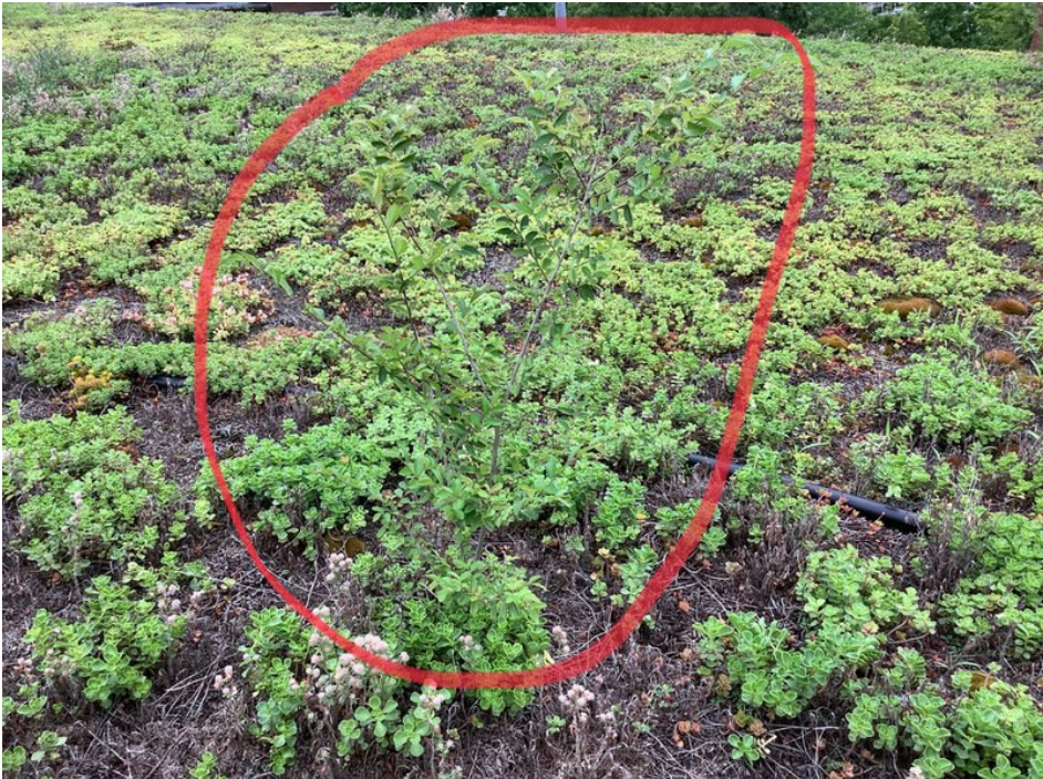
View of woody vegetation growing on the south end of the green roof.
