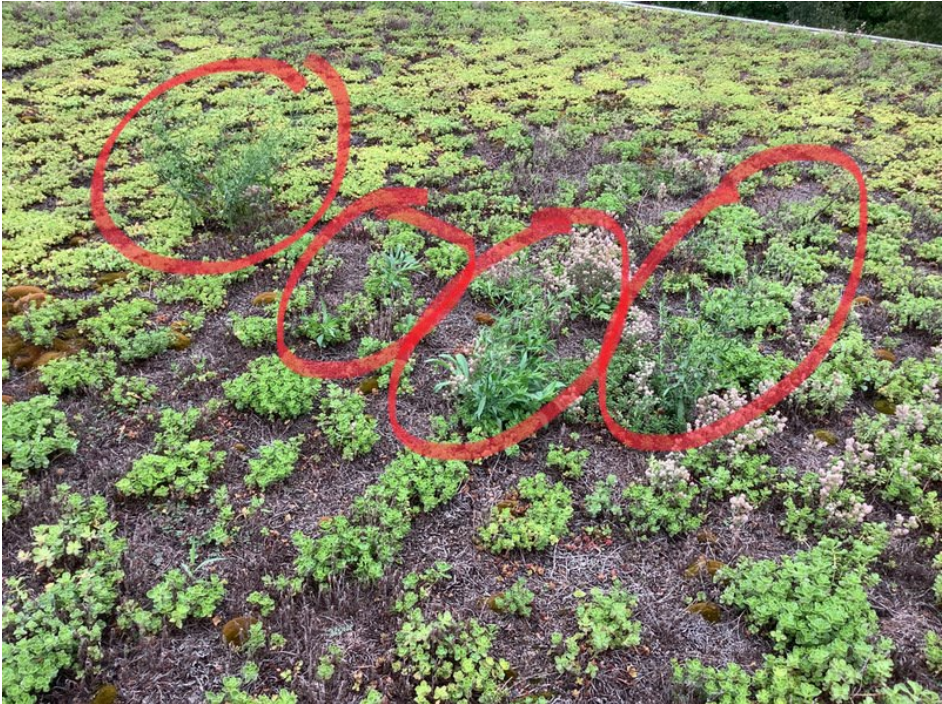
View of weeds growing on the south end of the green roof.
