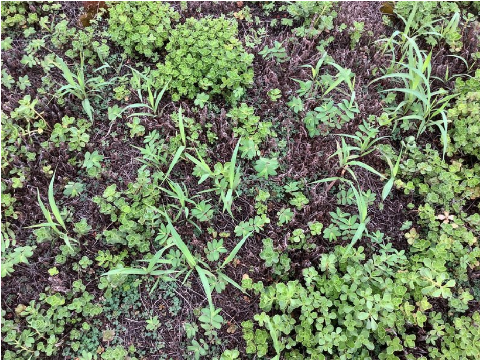
View of grass growing on the north side of the green roof.
