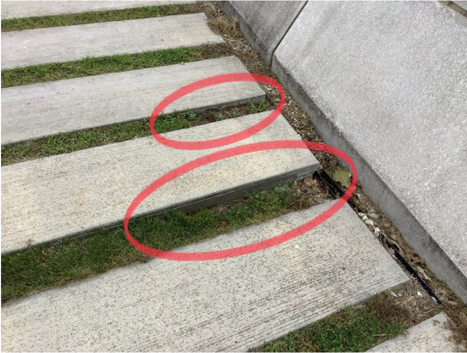
View of uneven pavers on the northwest section of the green roof (facing southeast).
