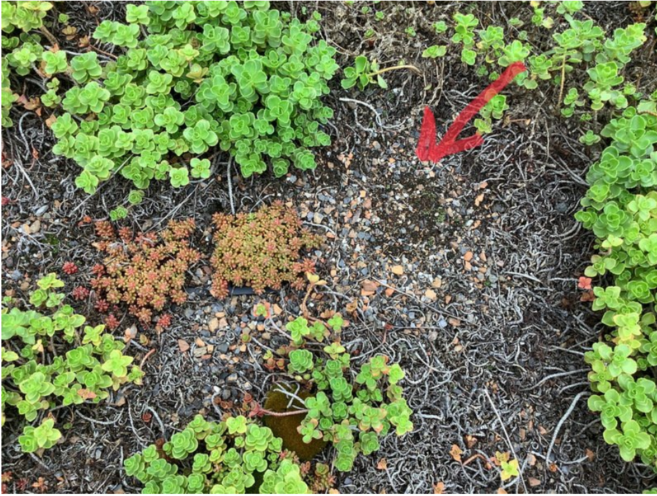
View of exposed soil media on the south end of the green roof.
