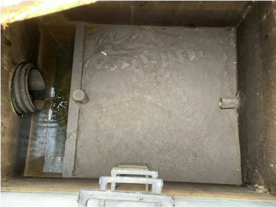
View of accumulated sediment in the west side of the sand filter.
