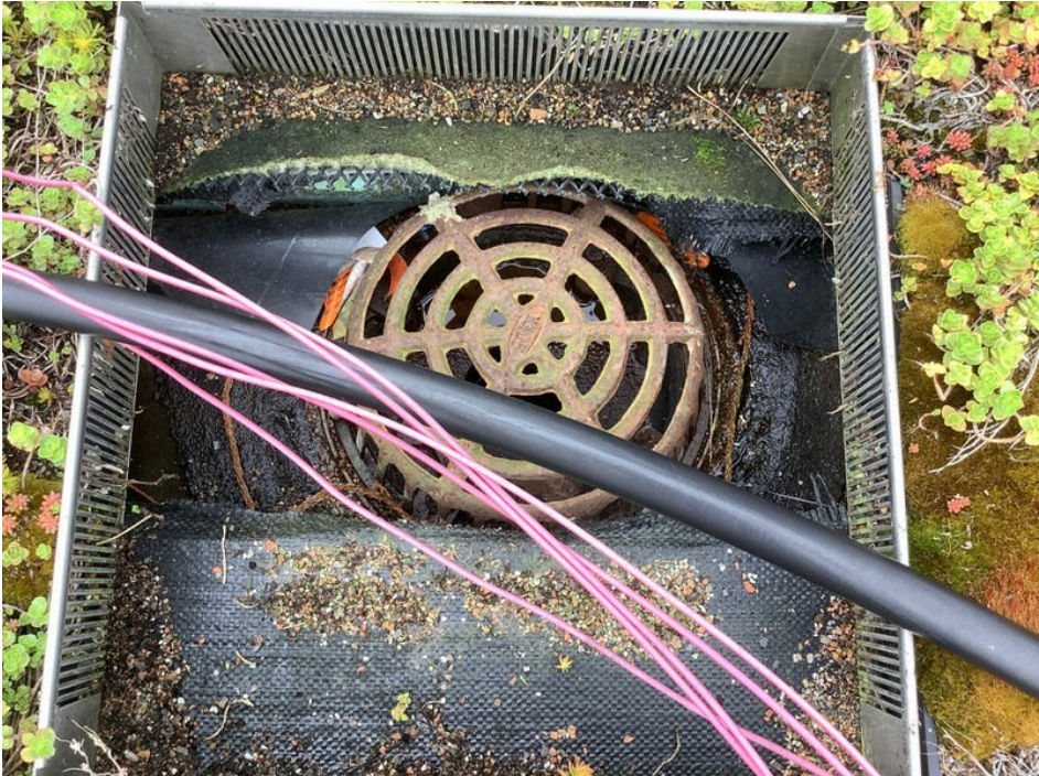
View of accumulated soil media in a roof drain on the south end of the green roof.
