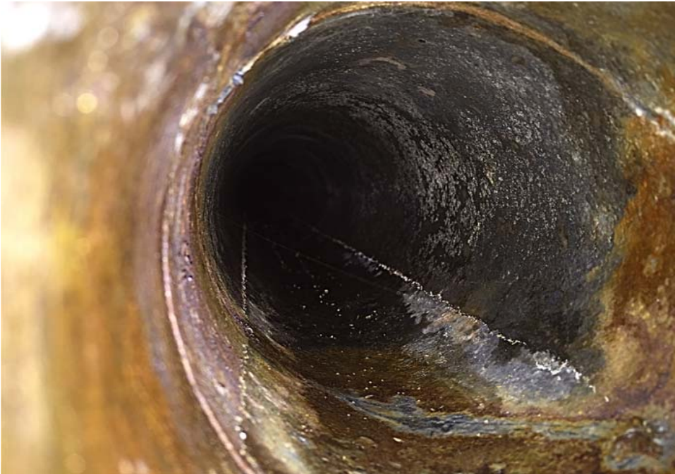
Four Inch Pipe Leading to East Tank
