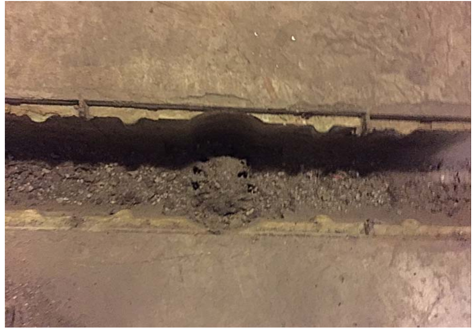
Trench Drain Before Cleaning
