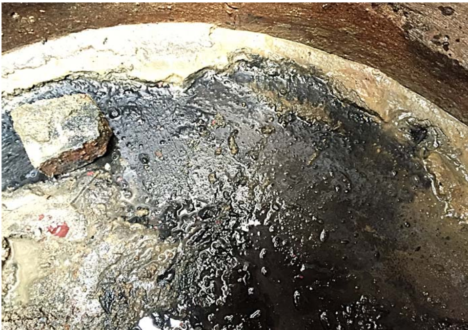
East Tank Bottom Following Liquid Removal. Sediment and Mortar Remains
