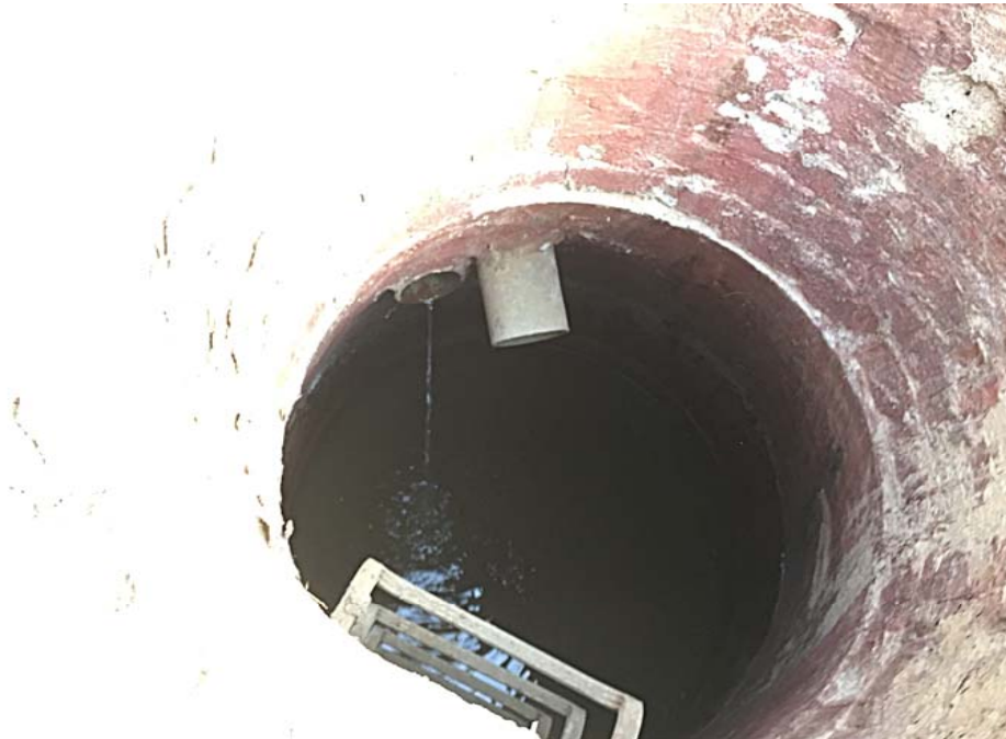
Flow Observed From Drain to Tank
