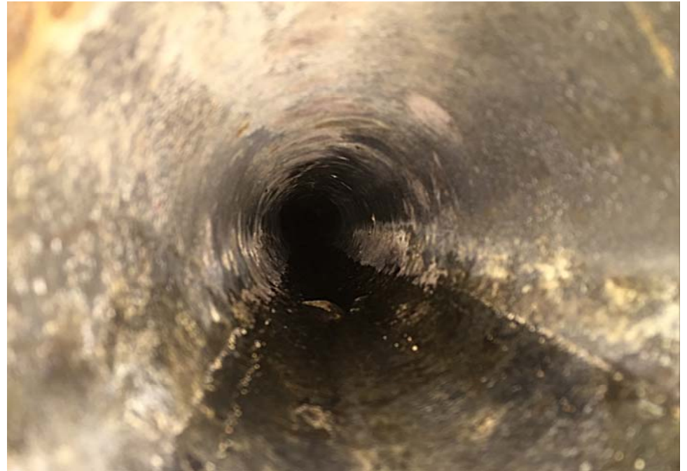
Four Inch Pipe Leading to West Tank
