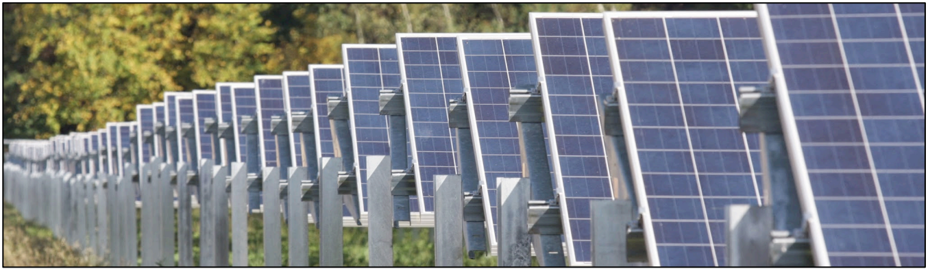
Skidmore's solar array
