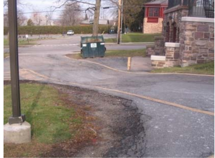
Driveway behind Hill Hall: Undulations in pavement, artificial low point corner of building
