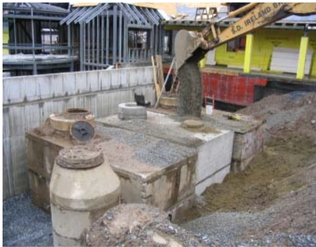
STORMWATER RETENTION TANKS
