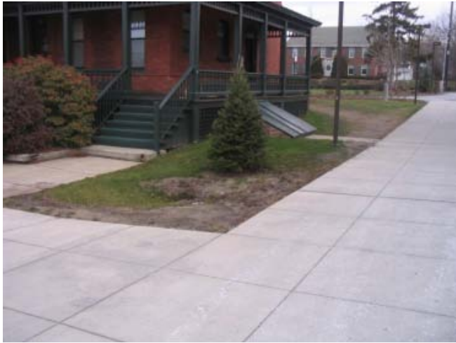
Ground area around/behind Aiken Hall -sediment build-up around CB, more foot traffic erosion
