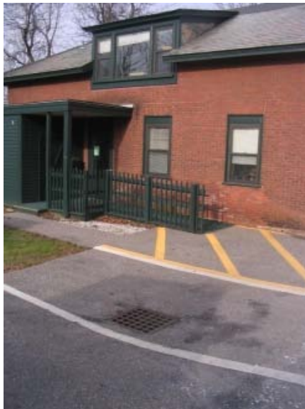
ARC building: CB w/ no apparent outlet; fills up during rain events, water seeps into basement
