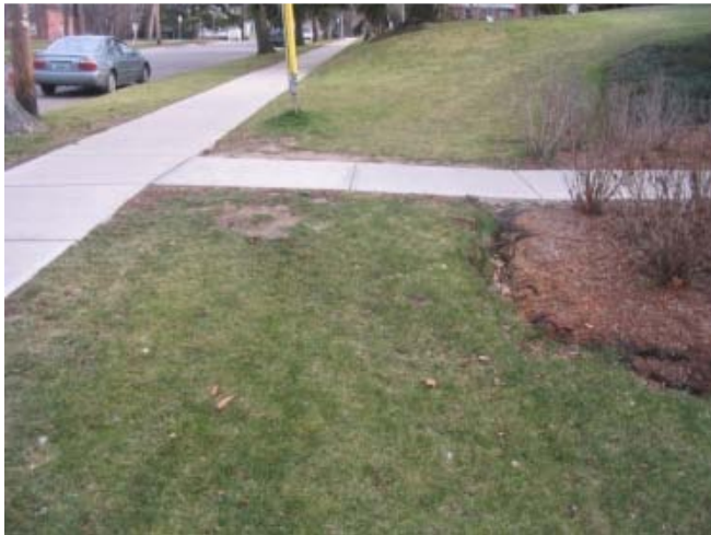
Entrance walk to S.D. Ireland Center, Maple Street side -Ties-in high point in city sidewalk causing storm water to flow toward building
