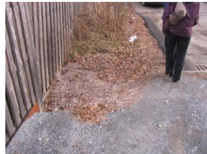
Break-away fence at end of Harrington Terrace: Build-up of leaves and sediment pushing up against fence, damaging hinges
