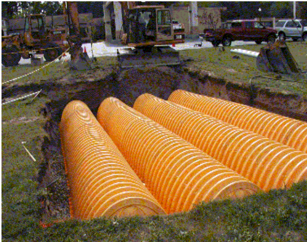
INFILTRATORS IN LAWN AREA
