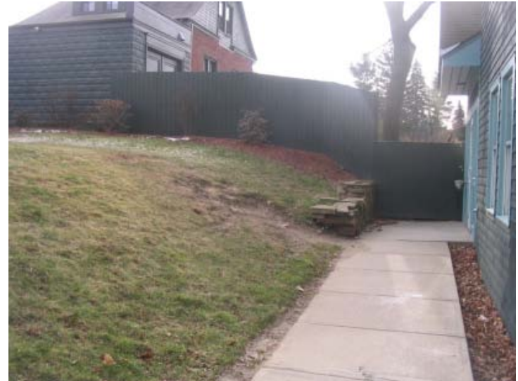
Behind Joyce Learning Center Slope erosion due to foot traffic
