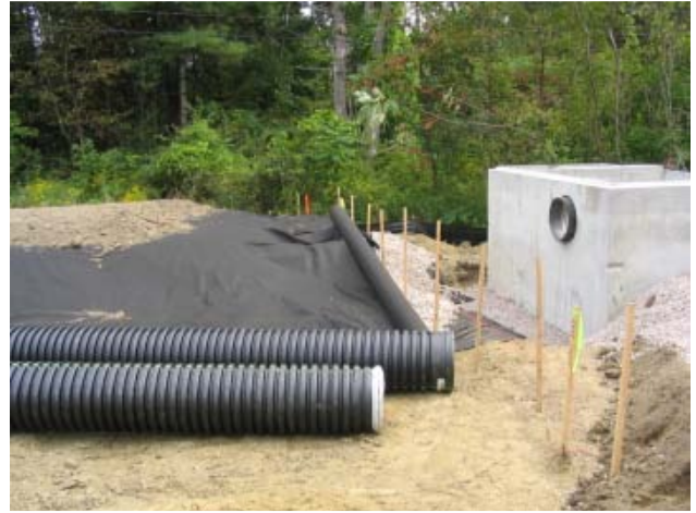
INFILTRATORS WITH TANK
