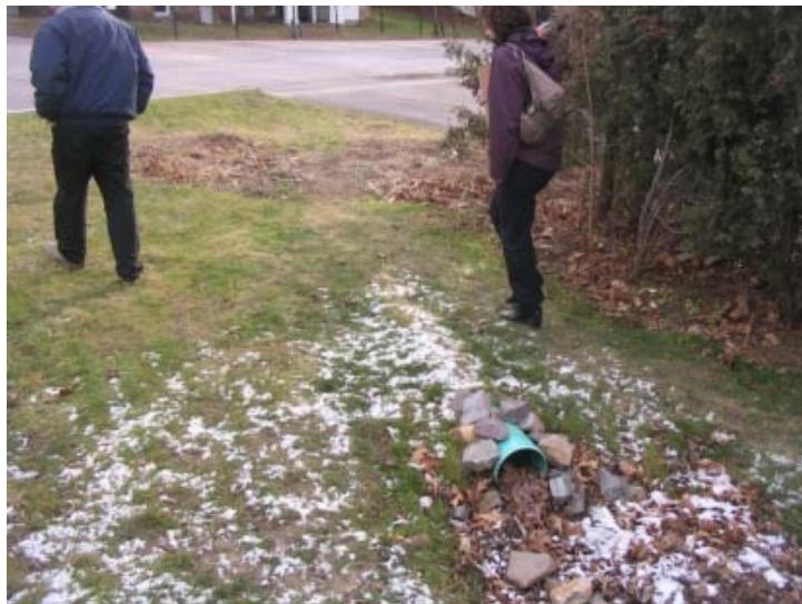
Discharge pipe to stone drainage swale
