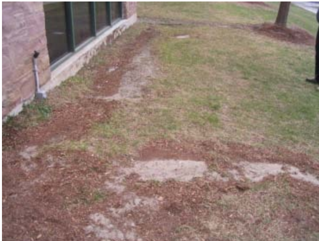
Ground area around Hauke Family Campus Center: Rooftop runoff causing erosion of ground area and sediment build-up
