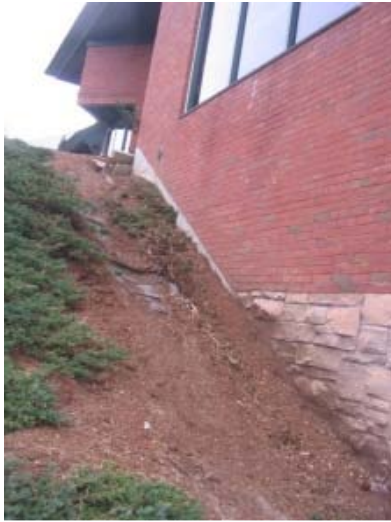
Slope beside Hauke Family Campus Center: Rooftop runoff/foot traffic causing erosion of slope
