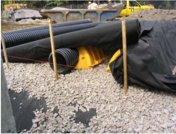
STORM WATER INFILTRATORS
