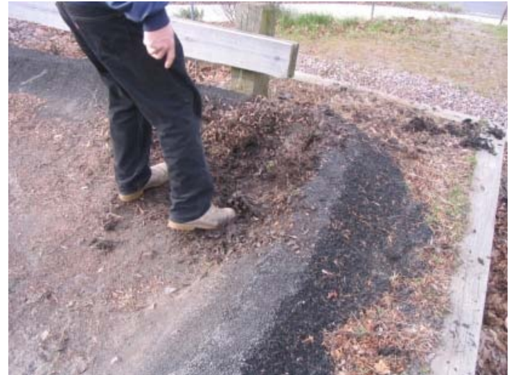
CB in corner completely buried by leaves and sediment
