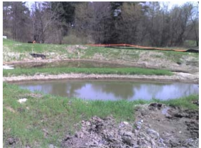
STORMWATER DETENTION POND
