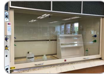
Figure 38: Another energy-saving opportunity is for campus users to appropriately shut fume hoods to minimize unnecessary ventilation
