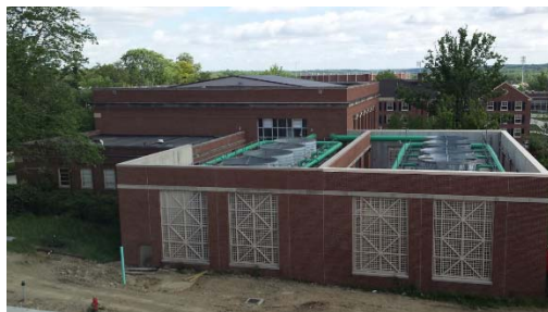
The North Chiller Plant.
