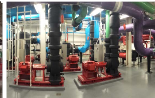
Pumps in basement of Western Geothermal Plant.
