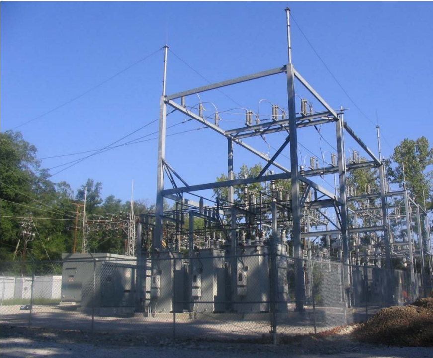
McGuffey Substation is located off of Rt. 73 by the Police Services Center.
