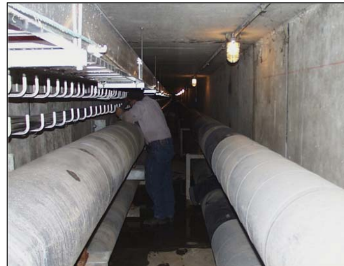
There are 5.4 miles of underground tunnels containing steam (lower right), chilled water (lower left), and communication lines (upper right) run throughout campus.
