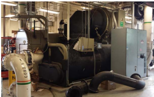
Centrifugal Chiller in South Chiller Plant.
