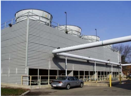
South Chiller Plant Cooling Tower cools water from 95°F to 85°F.
