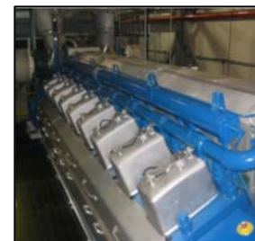
Bank of nine cylinders of the 18 cylinder engine.
