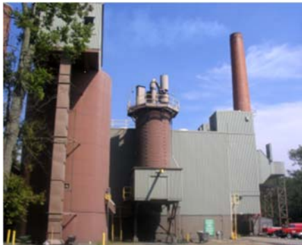
The steam plant produces steam year round for heating buildings, cooking in the dining halls, driving steam turbines that turn fans and pumps, humidification, processes in the chiller plants, and heating domestic water.
