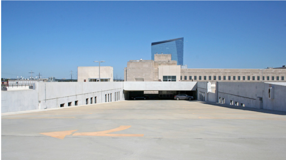
Top of garage
