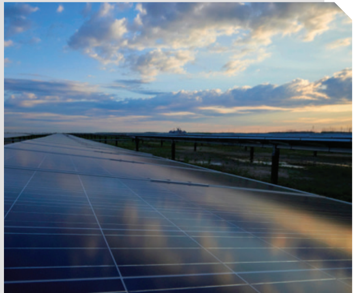
The Capital Partners Solar Project is a utility-scale solar farm in North Carolina.
