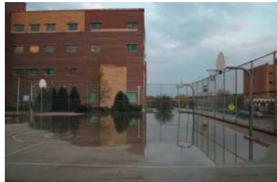
Existing ponding on the basketball courts after a rain. From Hartford Ave. School looking south to the Business School.
