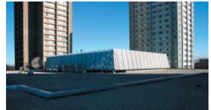
Commons roof and mechanical penthouse, looking north east. While a metal screen surrounds the penthouse, the structure is concrete.
