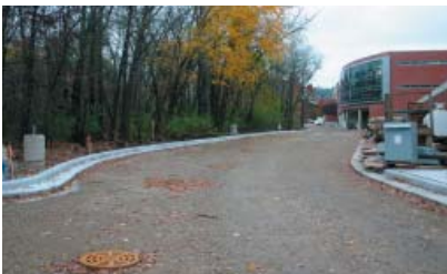
(below) The north service entry to the Pavilion, below which the storage pipe runs.
