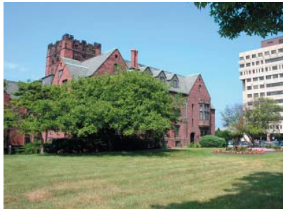
West facade, downspouts 12-16. Grounds clearly slope away from the structure and across open lawn.
