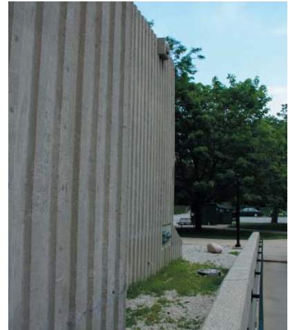
Scupper 7, showing the gravel filled area between the building and sidewalk that scuppers 7 through 9 drain into.
