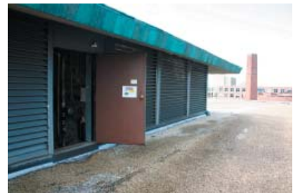
Service access door, north face of the lower hipped roof structure, housing the mechanical room
