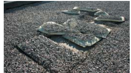
Commons roof insulation, disrupted and rising through the existing gravel ballast layer.
