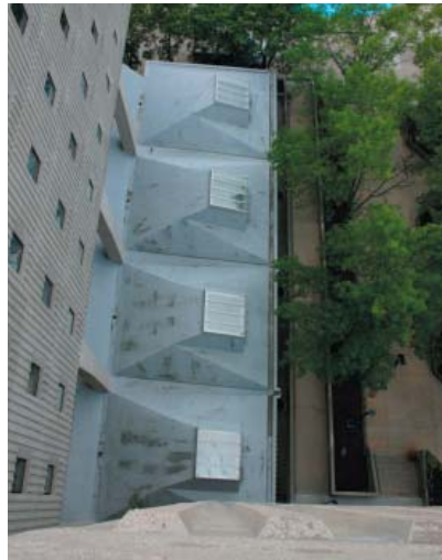
North lecture hall roofs from above. Each pyramidal form is capped by a skylight. The portions of the roof captured between the skylight and the mass of the building drain internally. The remainder of the roof area is collected in a gutter at the perimeter and allowed to spill out of the scuppers.
