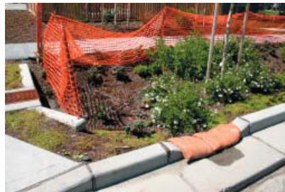
Hopes 6 Housing, Seattle. Mithun Architects, Designers and Planners. Curb cut draining to bio-retention area under construction.
