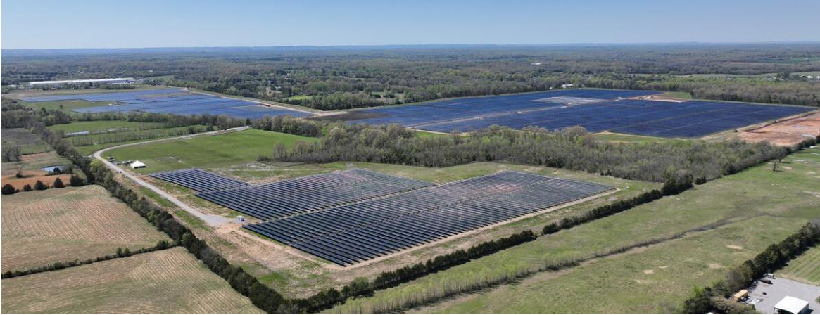
Figure 5 Vanderbilt I Solar Farm in Bedford County, Tennessee.
