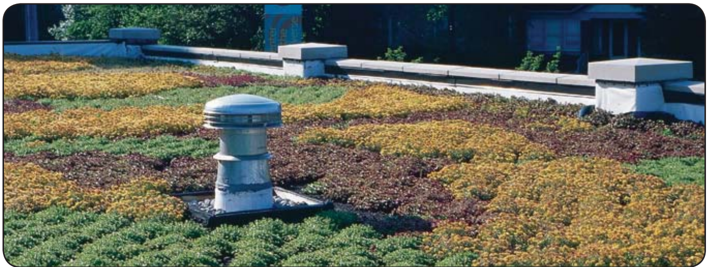
Fig. 4.28 Extensive Green Roof (LiveRoof, LLC www.liveroof.com )
