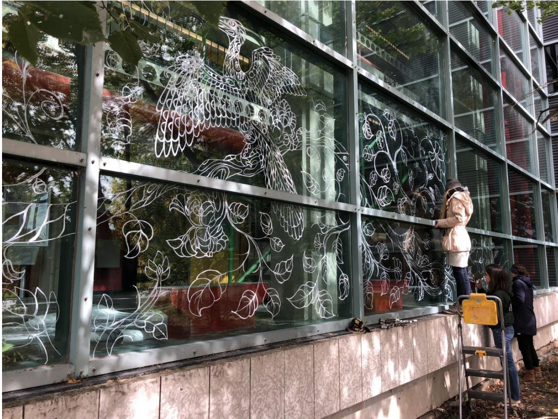
Photo 20: Vinyl decal artwork applied to Wallace Building windows to reduce bird collisions at Fort Garry Campus (Credit: University of Manitoba)
