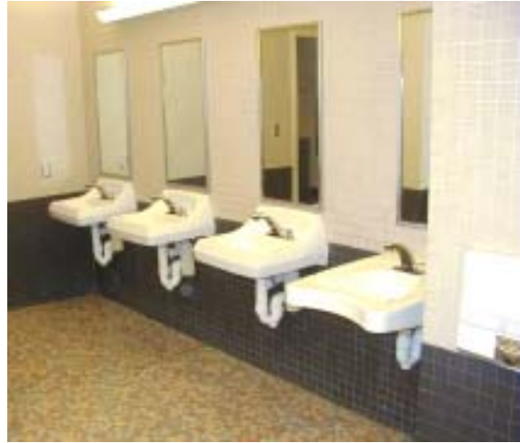
Rough service grade fluorescent lights, like the ones over these mirrors, last long, continue to look good, and do not suffer from cracks and other signs of abuse.
