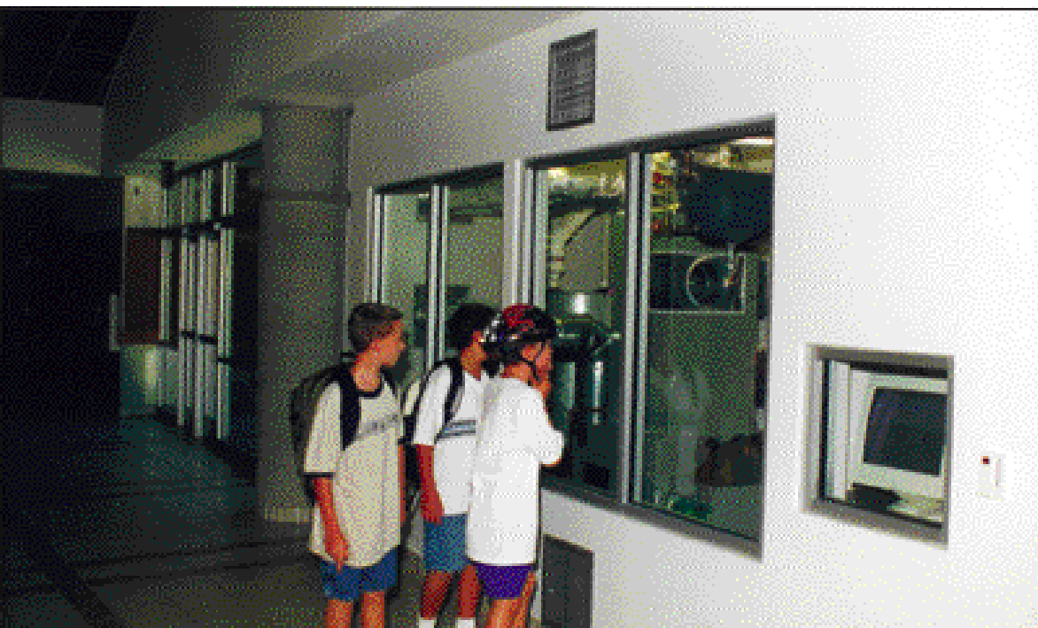
At Roy Lee Walker Elementary School, McKinney, TX, the energy-efficient mechanical system is exposed to serve as an educational tool for energy conservation.
