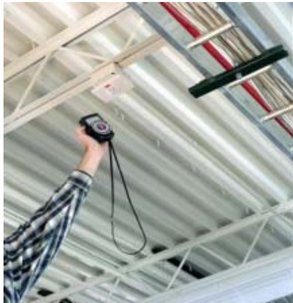
Light sensors, like the one being tested here, can dramatically affect both energy use and usability.
