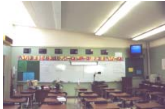
Automatic photosensor controls turn off first bank of lights next to skylight well. The light fixtures are arranged parallel to skylights to left and windows (out of picture) to right, while whiteboard is located perpendicular to windows and skylights.
