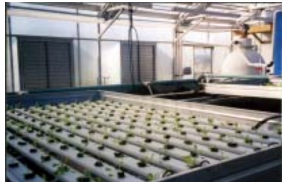
Geothermal heat pump systems reduce peak energy demand and reduce the heat island effect, since waste heat is returned to the ground instead of the outside air.
