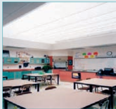
Figure S4.3 Classroom daylight monitors.
