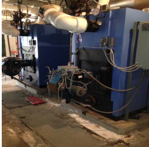
Figure 3.1: Two Unilux Heating Hot Water Boilers
