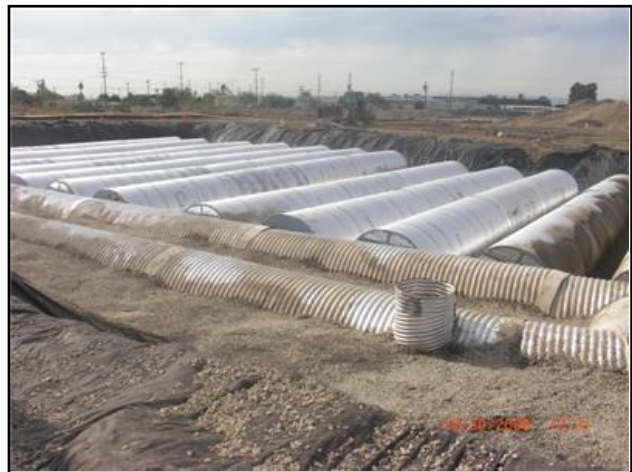
Underground Infiltration Units Lowe’s, Pacoima
