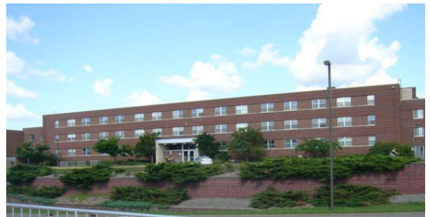
Retaining wall along Broadway Avenue in collegiate red. Scale is reduced by vegetation and blending color.
