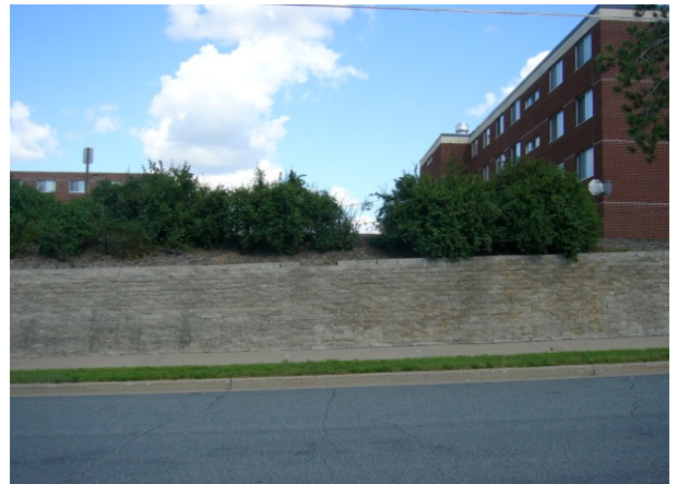
Retaining wall along 2 nd Street West is monolithic and harsh edge between north campus residence hall.
