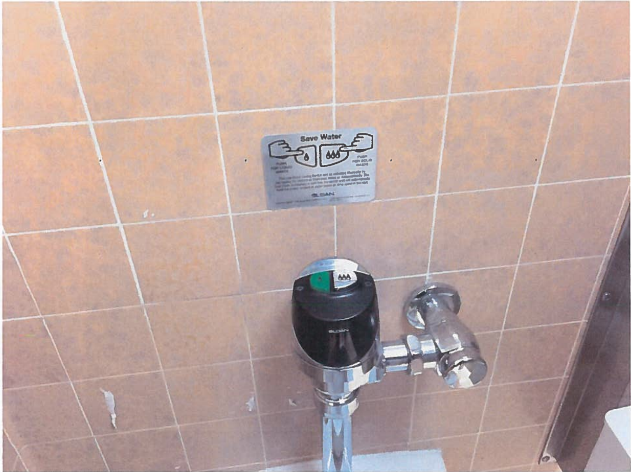
New toilet fixture has a sticker that shows how to reduce water usage when flushing.
