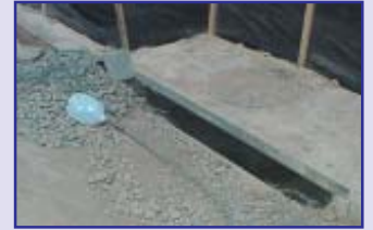
Failed Inlet Protection
