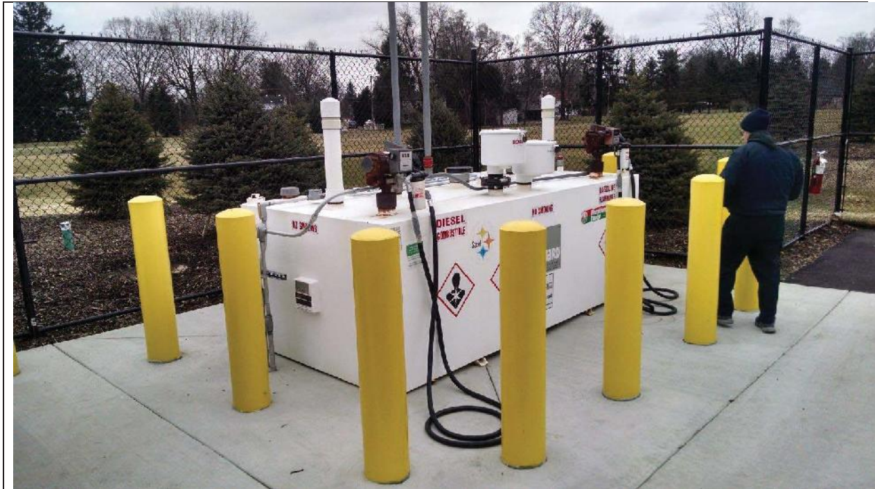
Fuel Pump Station
