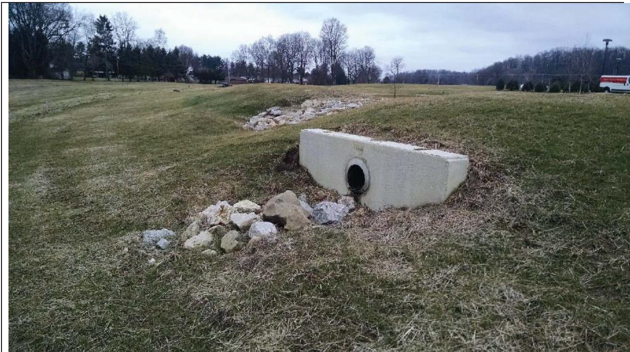
Stormwater Infiltration Basin – Facility Outfall
