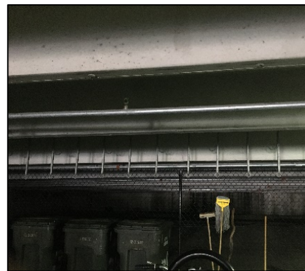
Figure 3. The ceiling bike hooks are in the George Street Parking Garage, but are not utilized and are obstructed
