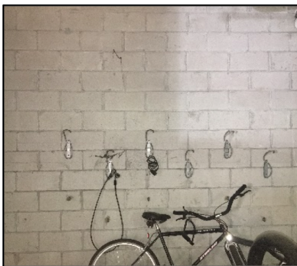
Figure 2. The bike hooks are in the George Street Parking Garage. These bike hooks are not being utilized now
