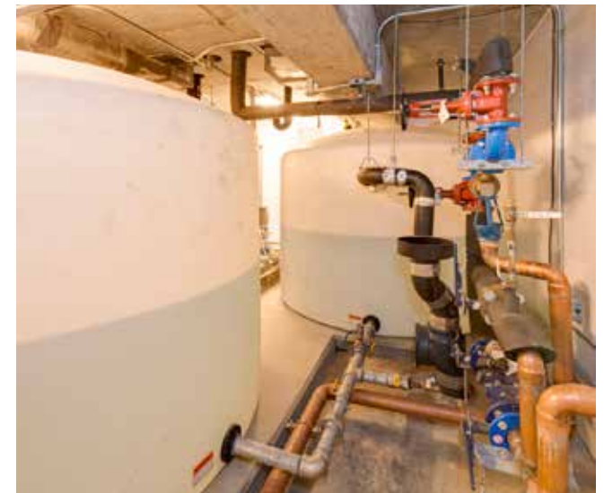
Figure 5-28 Rain Water Harvesting System, Brock Center, Virginia Beach, Virginia
