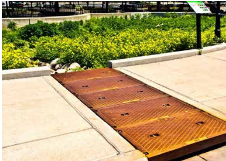
Figure 5-50 Stormwater Flume to Rain Garden with a Sidewalk Plate
