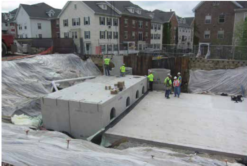
Figure 5-45 StormTrap Underground Detention Chamber, Lot 45
