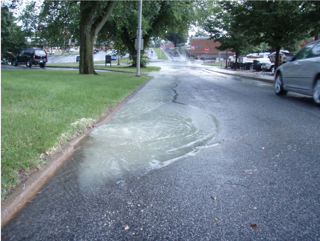
Figure 6.v. Surcharging of Mckean Road Inlet for a Moderate Rainfall Event
