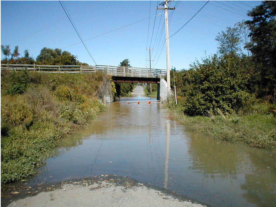
Figure 4.k. Flooding of the Corl Street Underpass in West Campus
